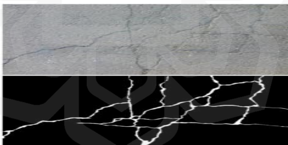
Figure 2.5. Crack Segmentation (P. Li et al., 2022a)
