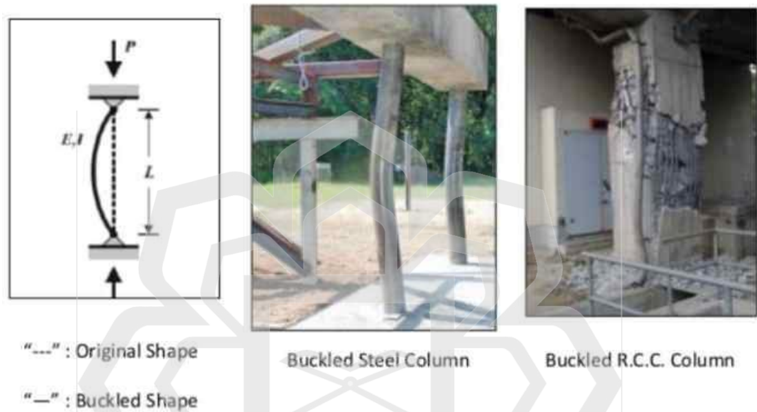
Figure 2.5. Buckled steel column.
