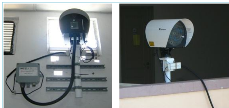
Figure 3.4. Installation site of FSO links head at location A and location B
