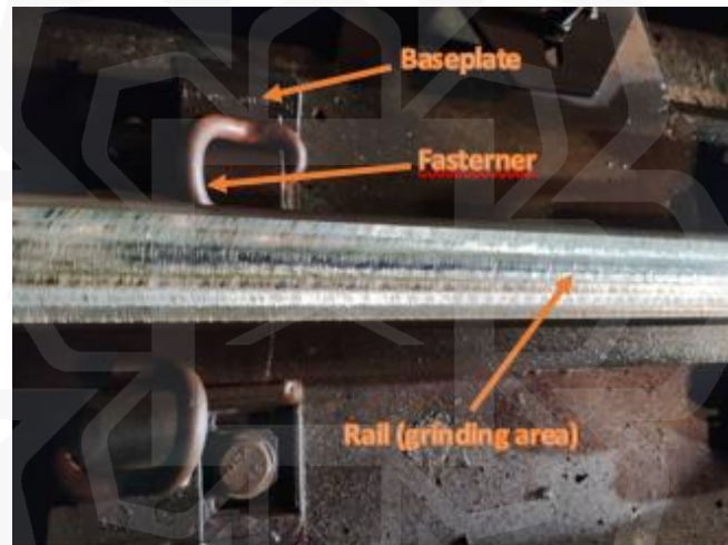
Figure 3.11: Rail track condition after rail grinding process.
