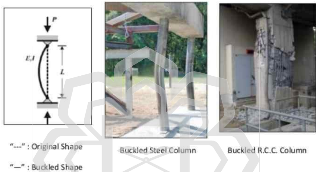
Figure 2.5. Buckled steel column.
